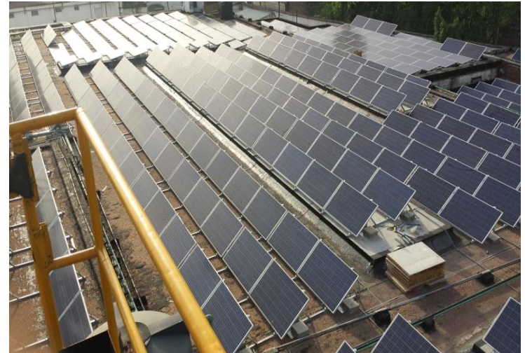
ITC - 2MWp+ (Various Locations)
