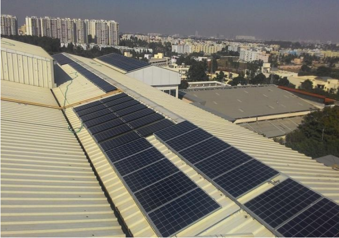
Infosys - 300kWp + 3 MWp
