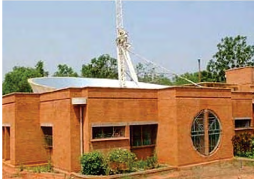
Solar Parabolic Concentrator installed on top of Kitchen
