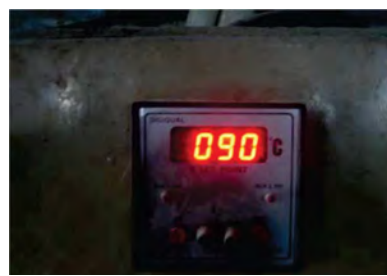
Temperature sensors on the duct
