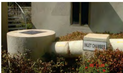
Inlet Chamber from the Pre-digester
