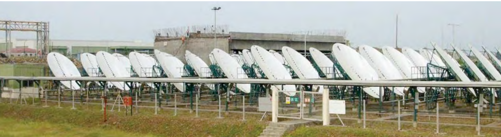
SolPac-D160 (Thermax) installed at MVML, Pune
