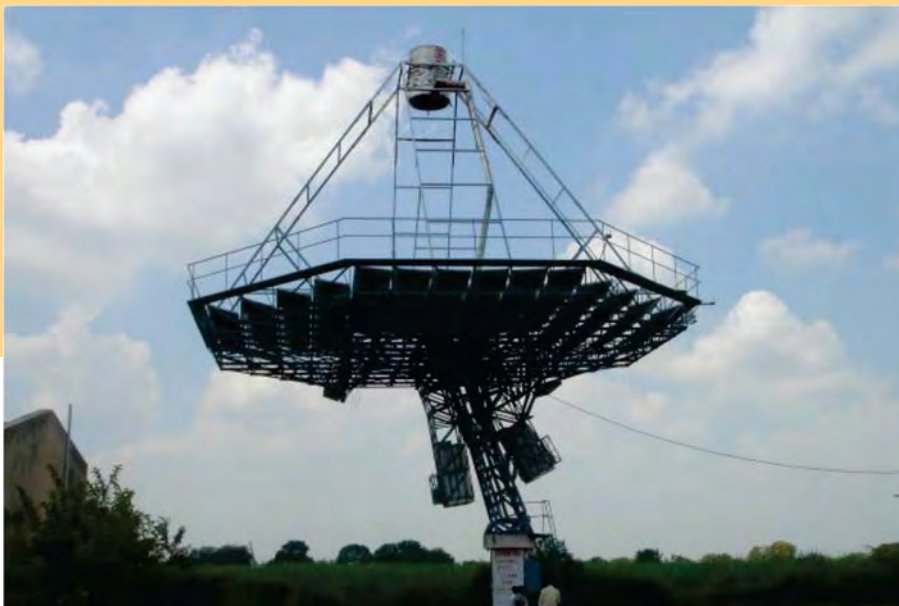
Solar Parabolic Concentrator installed at Mahanand Dairy Unit top of Kitchen
