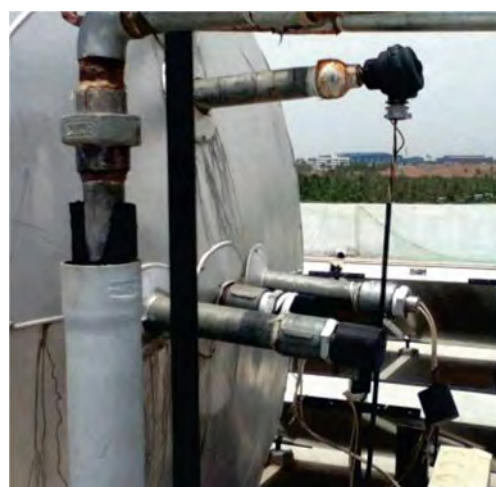
Insulated Solar Water Tank and pipelines
