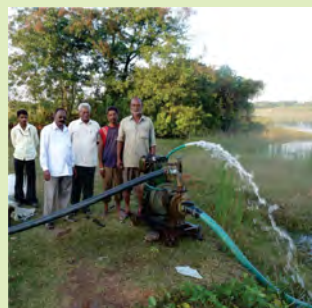
Diesel fired irrigation pumpsets
