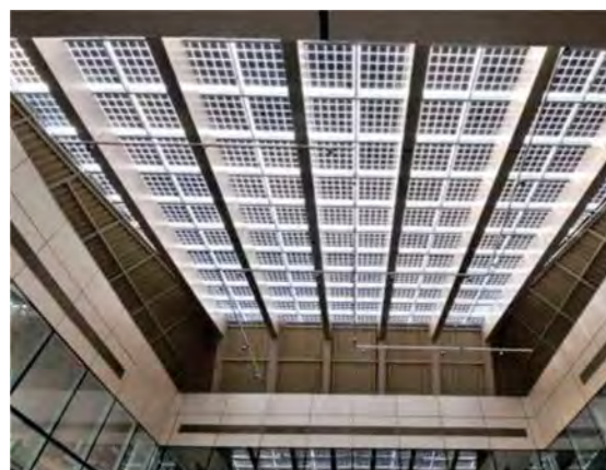
13.5 kW Bi-PV systems integrated with the roof
