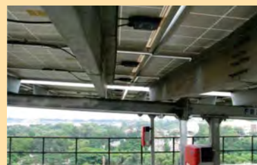
String inverters installed under the panels
