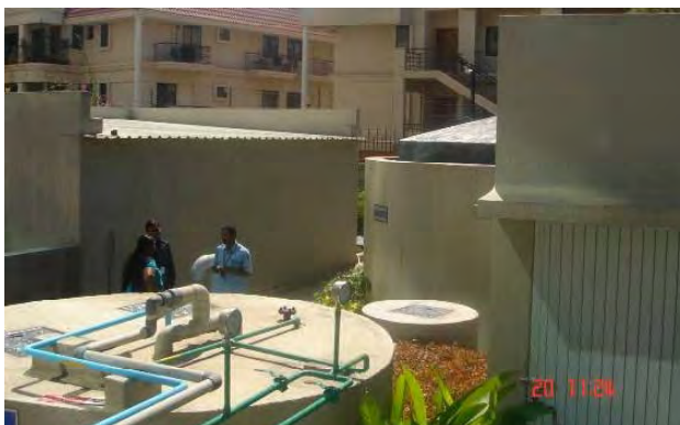
Hot water and gas pipelines to the Pre-digester
